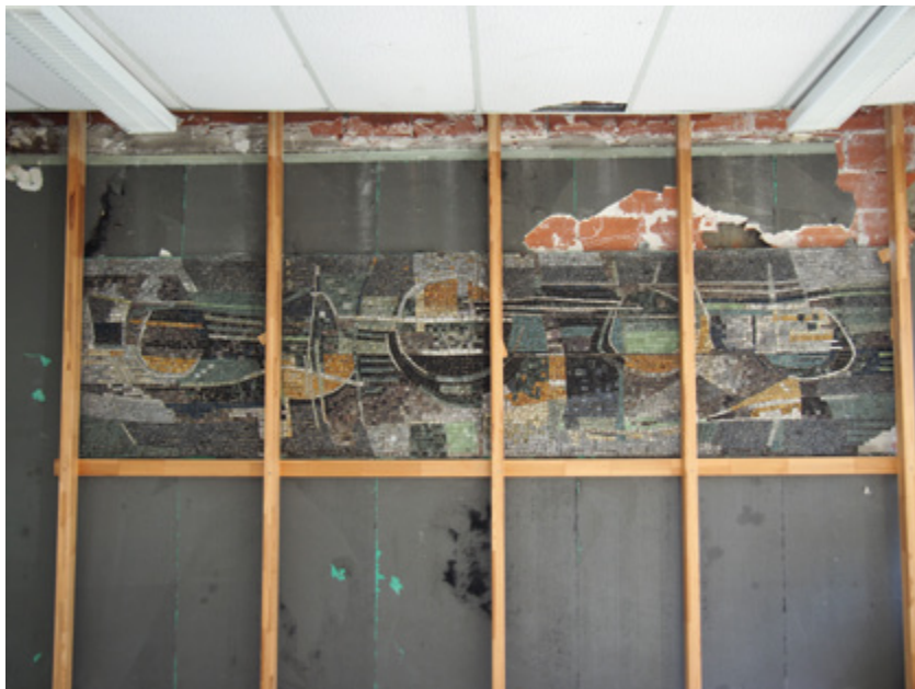
Picture1. The green mosaic before protection and removal of its old wall. (Photo: Astrid Maréchaux)
